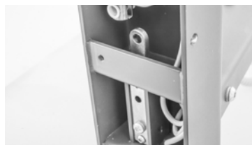
View after disconnecting actuator
